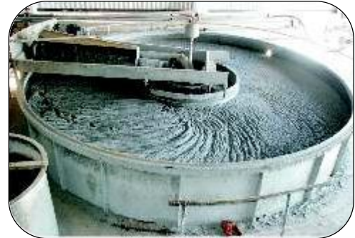
Effluent Treatment Plant
