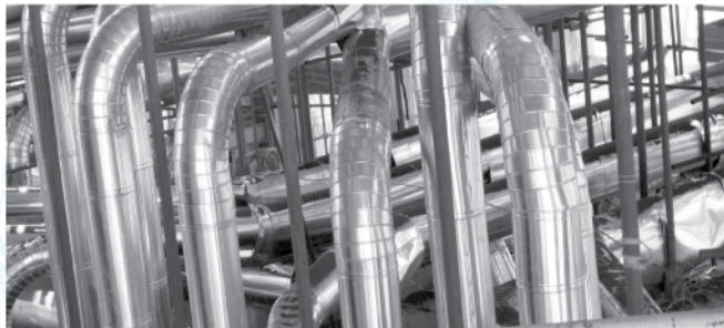
Rockwool Insulation & Refractory
