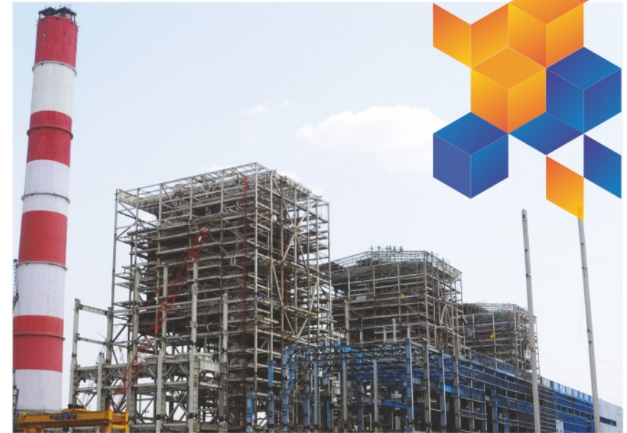
Erection & Associated Works of Boiler & Auxiliaries & TG Auxiliaries for Unit 1 & 3 for 3X660 M.W. Tiroda Thermal Power Project, Adani Power Maharashtra Ltd., Tiroda, Maharashtra
