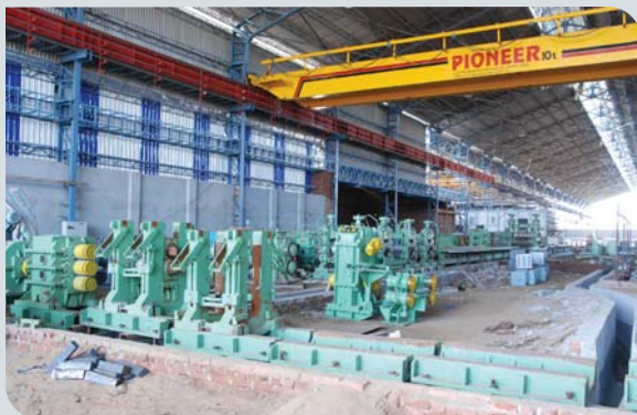
ROLLING MILL AREA
