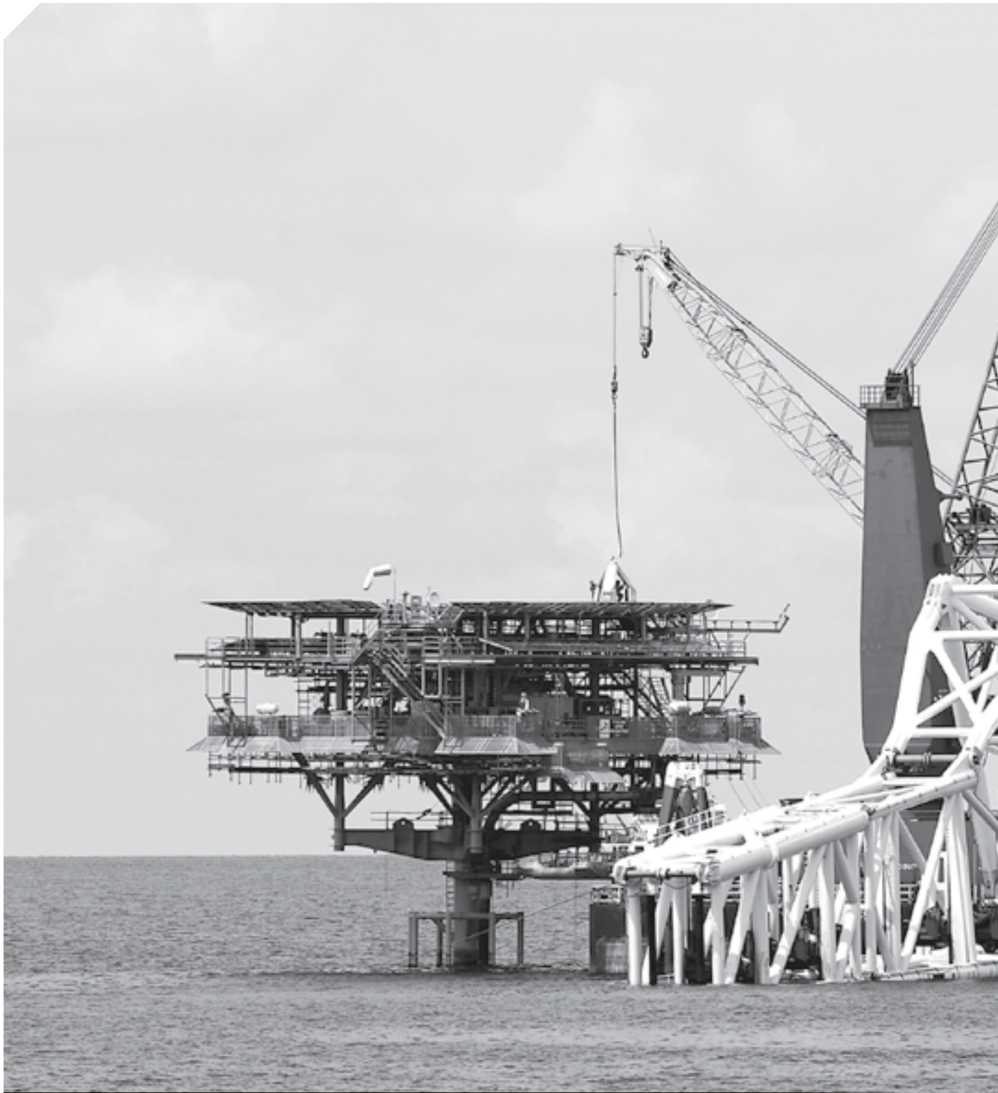
PUNJ LLOYD'S PIPELAY BARGE, KUBER AT WORK ON THE OFFSHORE PLATFORM PROJECT FOR PERTAMINA, INDONESIA
