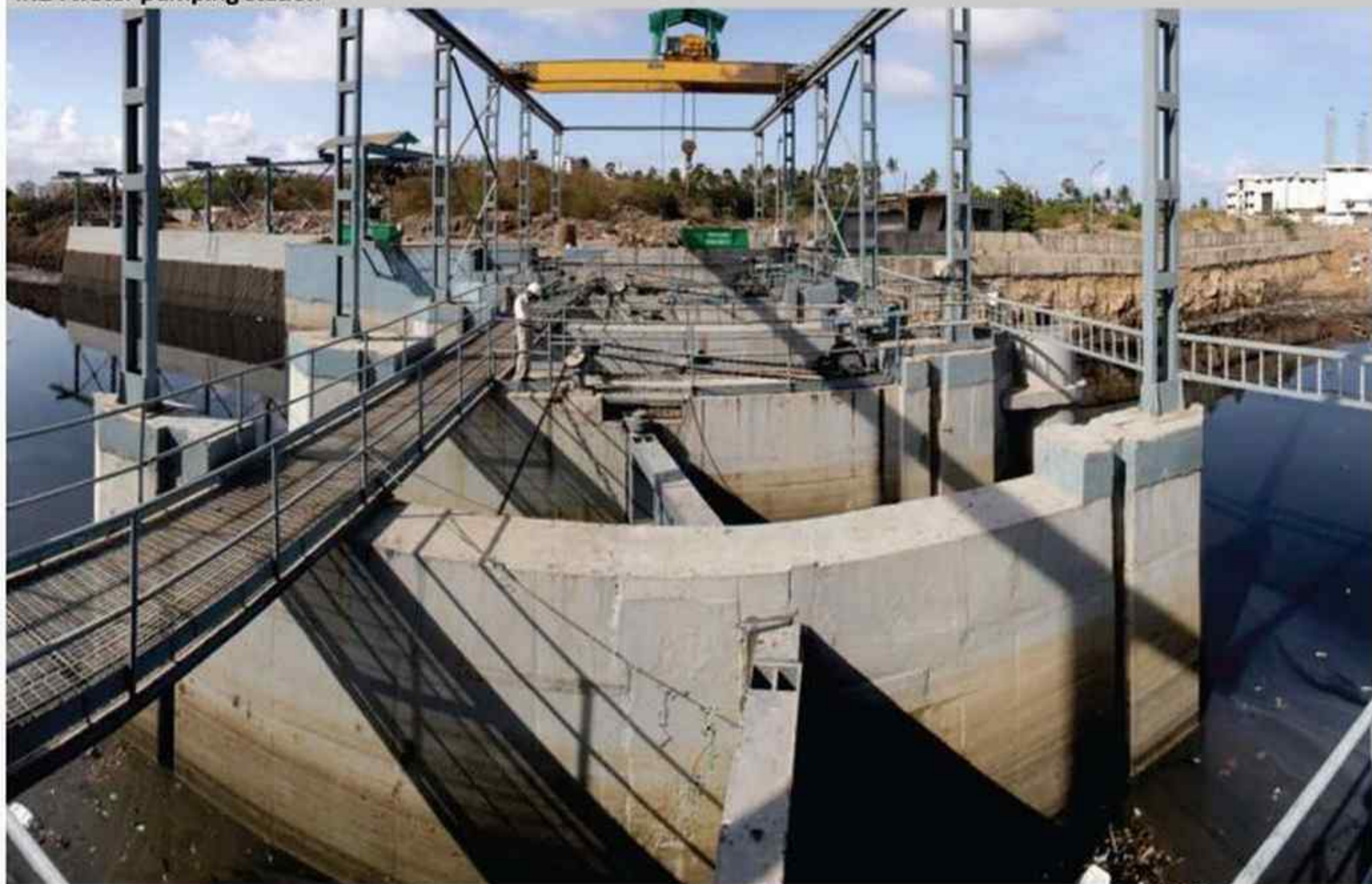
IRLA water pumping station
