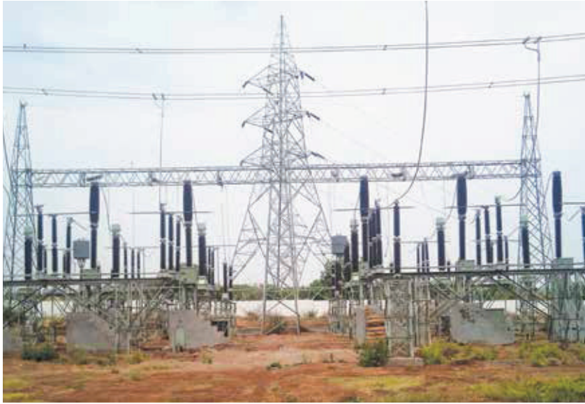
▶ 132/33 kv substation in Andhra Pradesh
