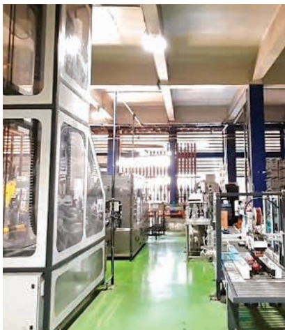
Productivity improvement at Silvassa: Installation of an advanced filling line to enhance our responsiveness and capability to meet fluctuating demand service needs for OEM and other companies more efficiently
