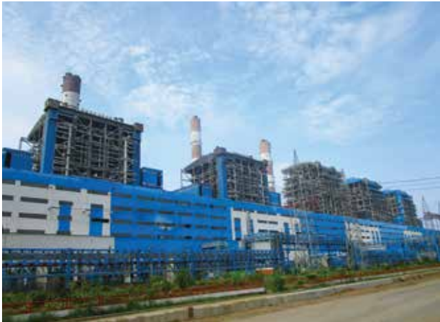
3x660 MW Stage-I STPP Boiler, Barh
