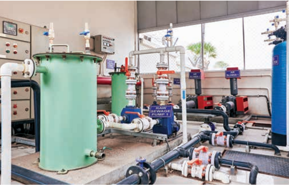
Sewage Treatment Plant (STP)
