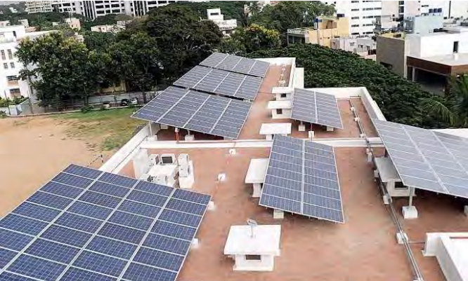
Installed Solar Panels at Surangi Unit to reduce Carbon Emissions per month
