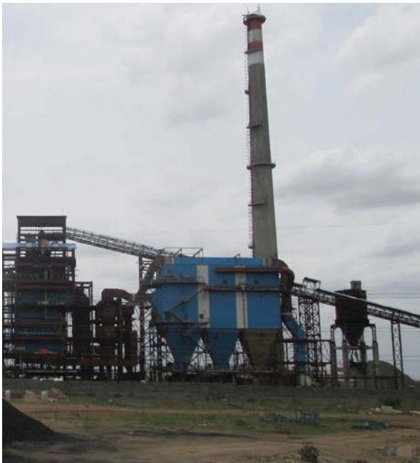
Captive Power Plant - Muktyala
