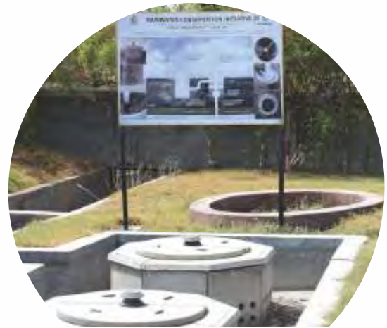
RAINWATER HARVESTING AT KALOL PLANT
