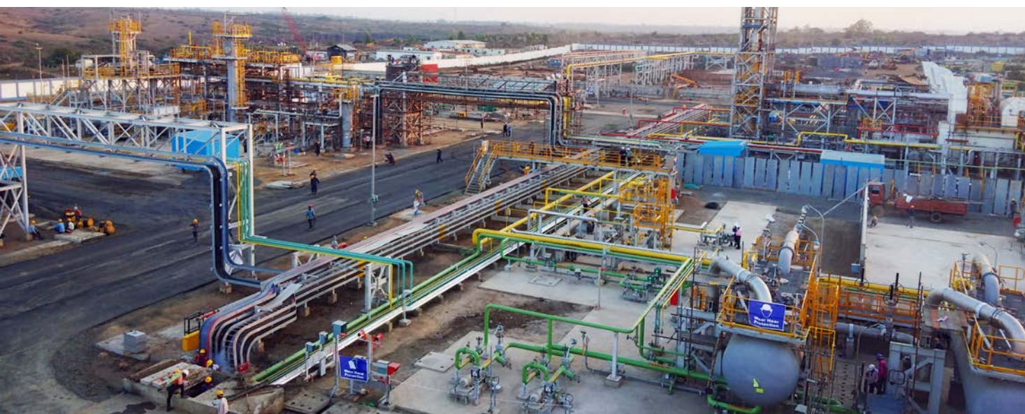
Coal Bed Methane Project (Phase II) for Reliance Industries at Shahdol, India
