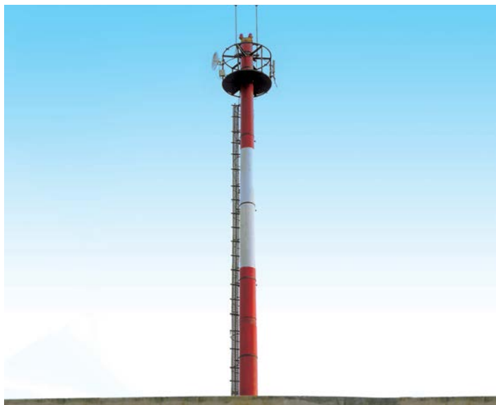
Early Warning Dissemination System, Odisha
