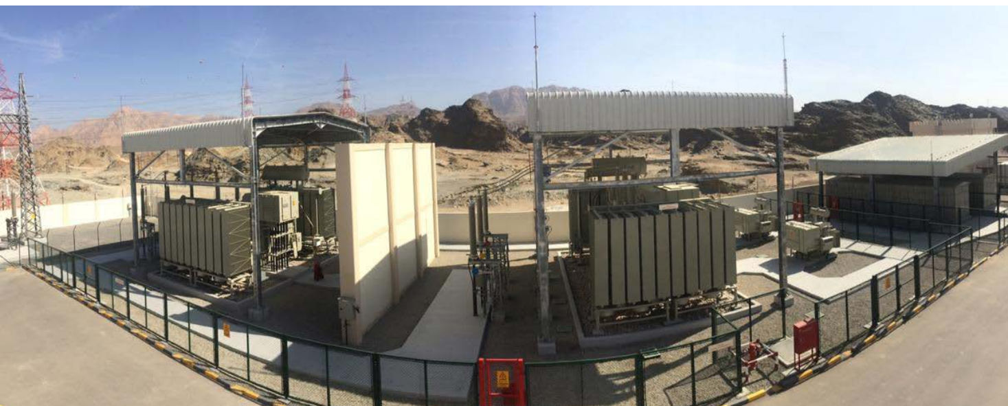
132/133 kV Grid Station at Ghala Heights, Oman
