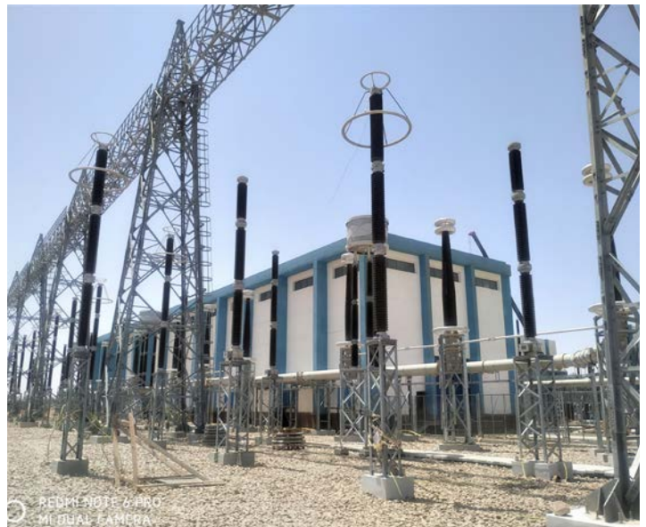
500/220 kV S4 Ras Ghareb Gas Insulated Substation, Egypt
