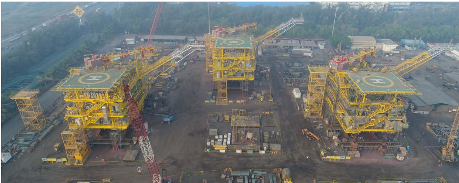
Three Gas Production Deck Modules (PDMs) for Saudi Aramco, ready for dispatch from LTHE's Modular Fabrication Facility at Hazira, India
