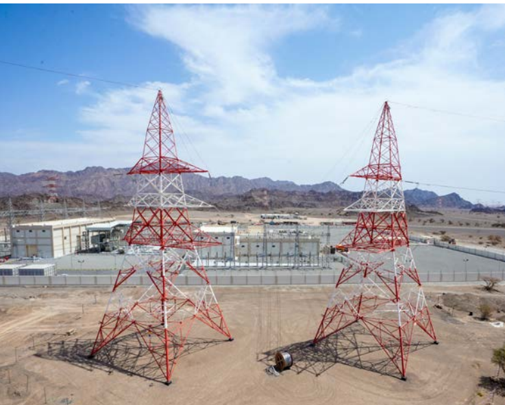
400/132 kV Grid Station at Qabel, Oman
