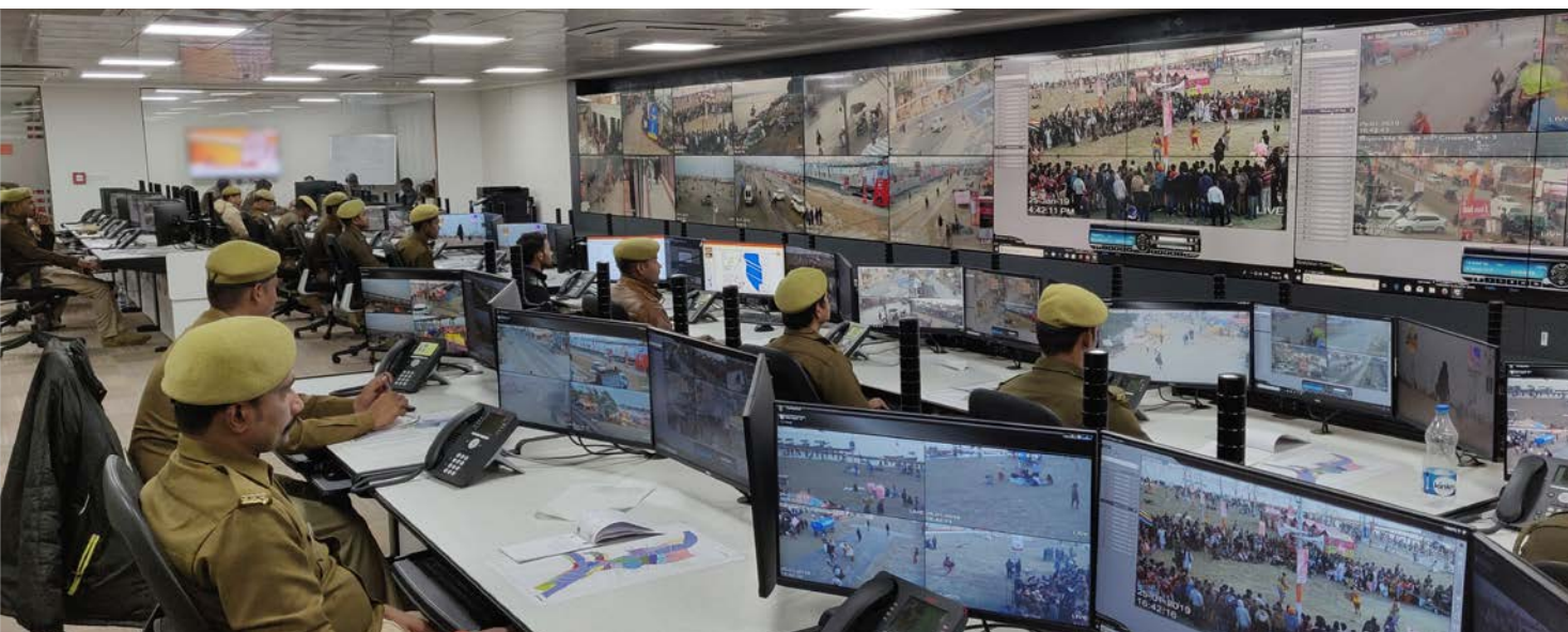
Command & Control Centre, Prayagraj
