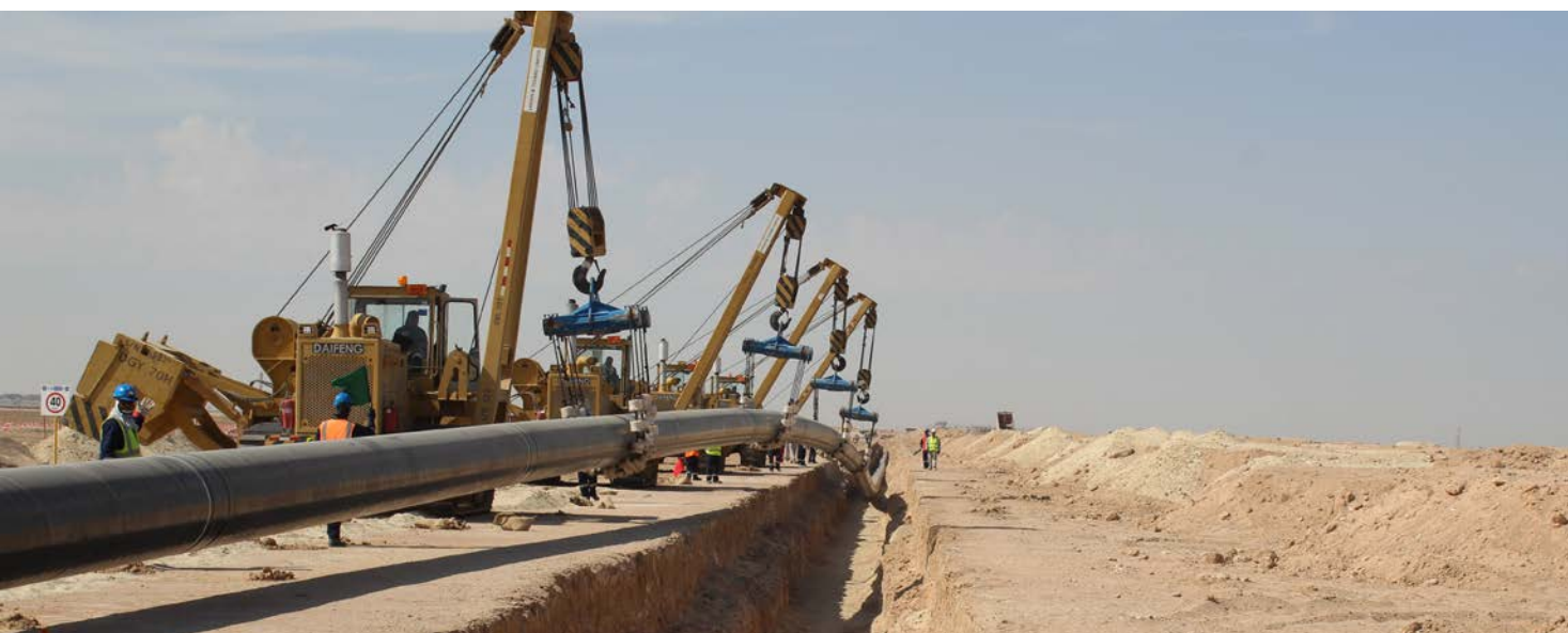
Lowering of new strategic gas export pipeline (Size: 30" / 40" x 146 km) from North Kuwait to Mina Al-Ahmadi for Kuwait Oil Company
