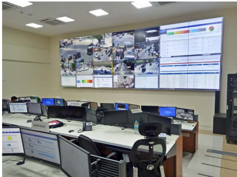
City Command & Control Centre, Vadodara Municipal Corporation
