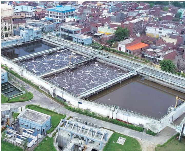
Moradabad Sewerage Treatment Plant, Uttar Pradesh
