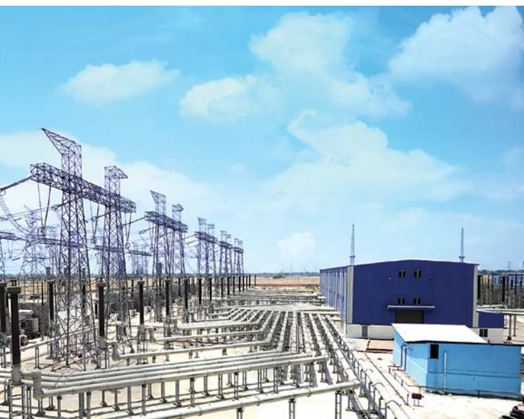
765 kV Gas Insulated Substation, Varanasi, Uttar Pradesh
