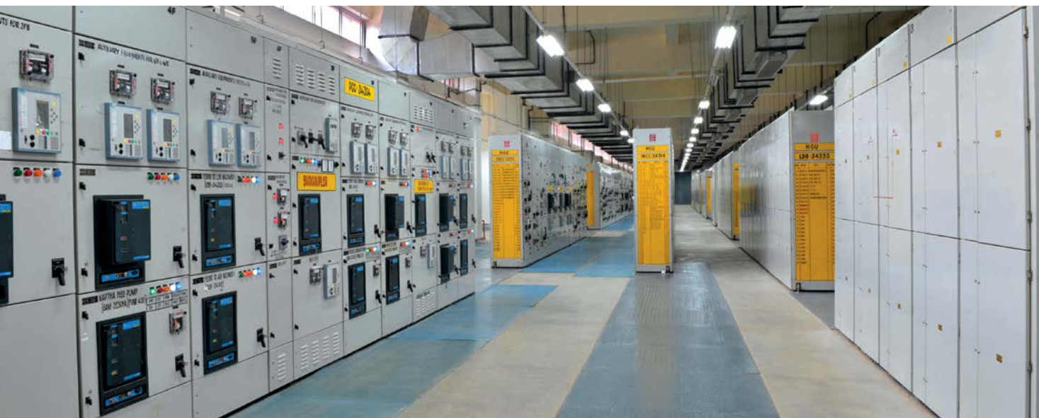
Control panels at MRPL
