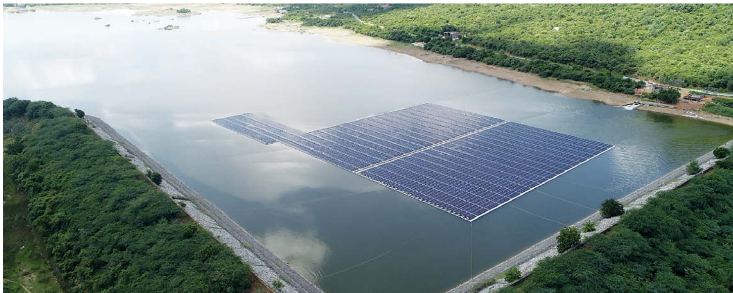
Floating Solar Project, Tirupati, Andhra Pradesh
