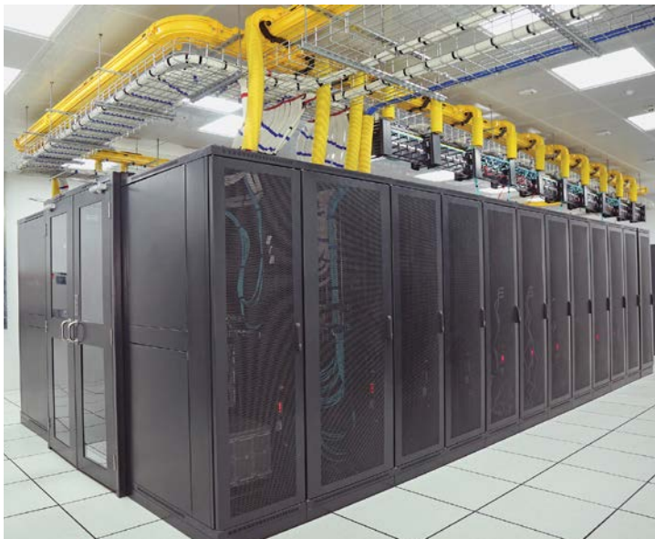
Data Center, Hyderabad
