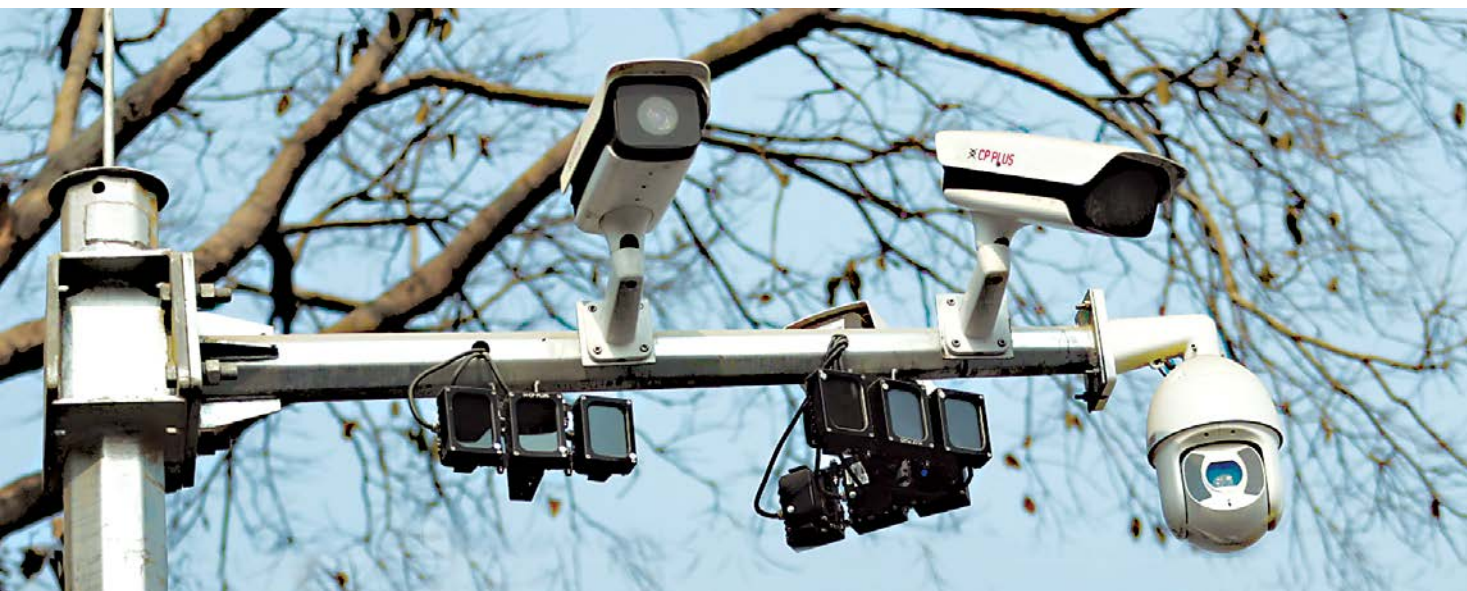
Surveillance cameras installed at Prayagraj
