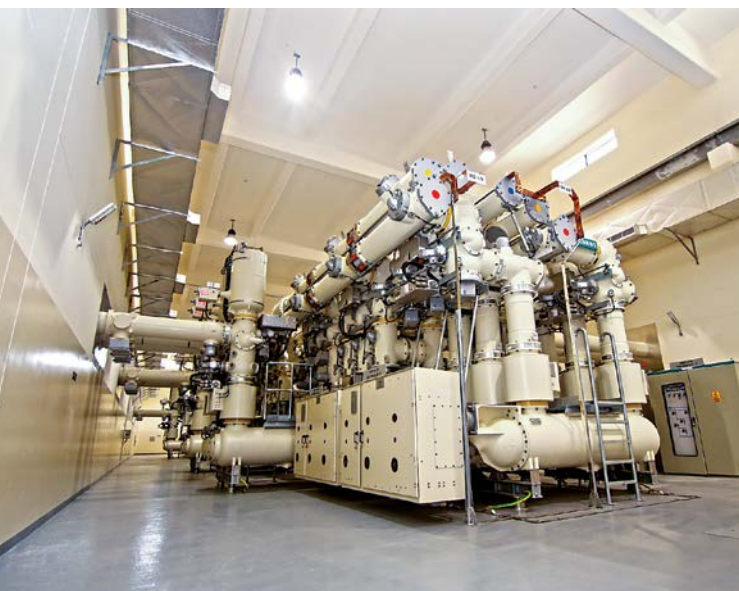
400 kV Grid Station at Misfah, Oman
