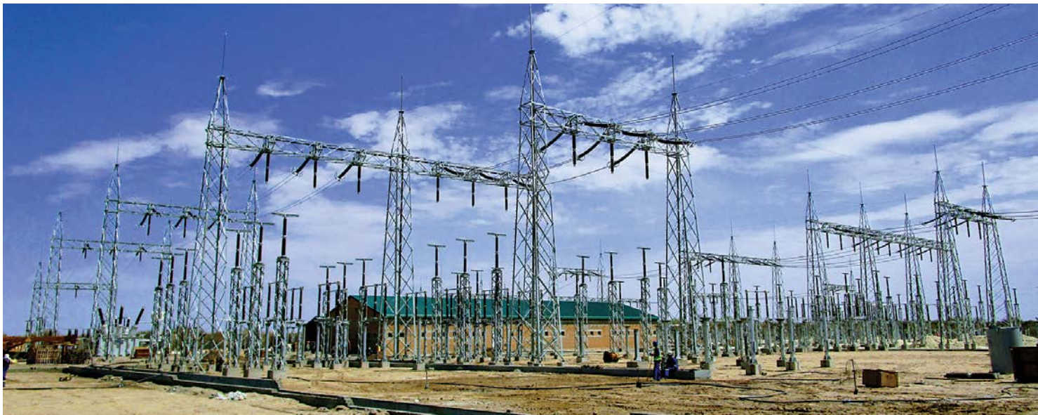
400/220/132/33 kV Substation, Mawana, Botswana
