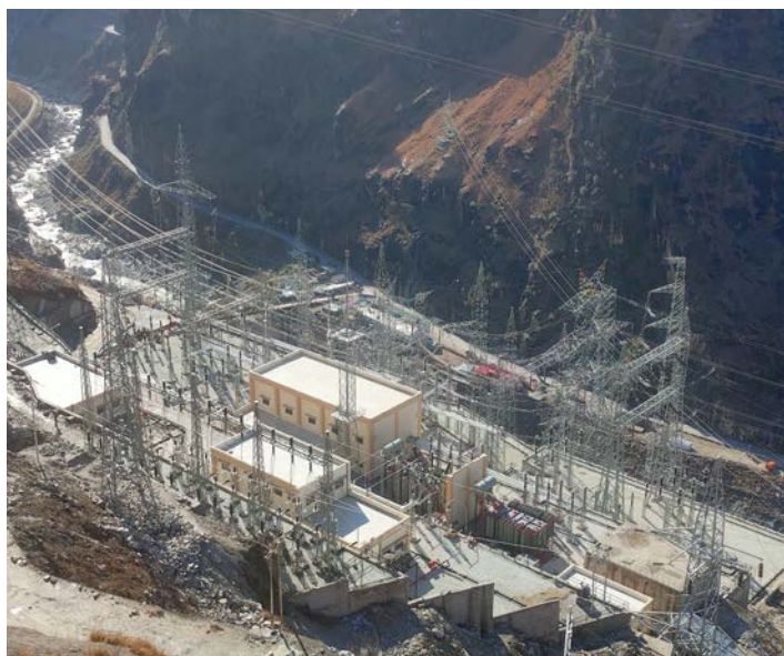
400/220/66 kV Substation at Wangtoo, Himachal Pradesh
