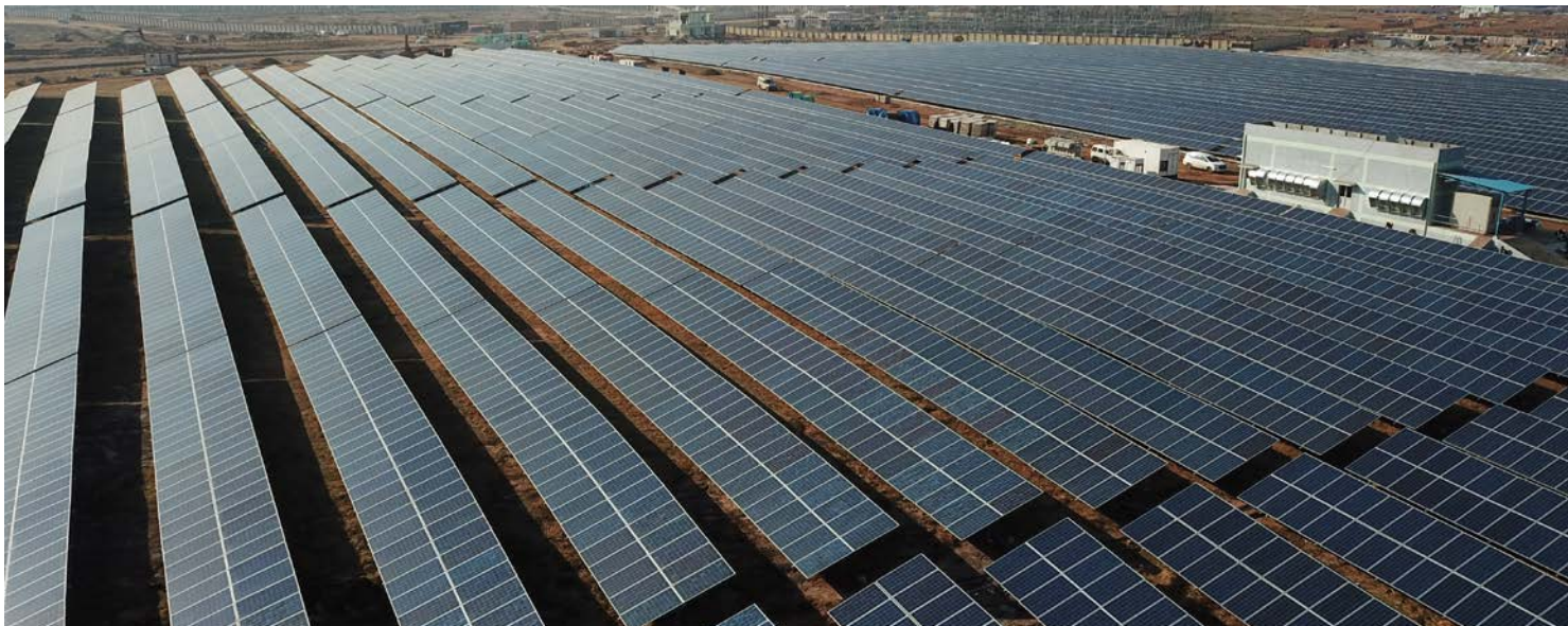
250 MWp Solar PV Plant, Madhya Pradesh
