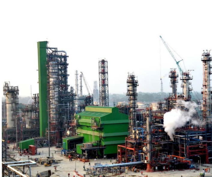
INDMAX FCC Unit including LPG Treatment Facility for IOCL, Bongaigaon, India
