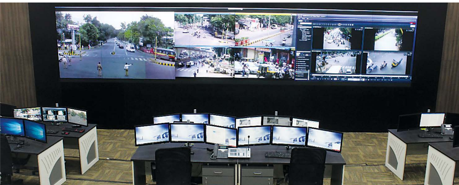
City Operation Centre, Nagpur
