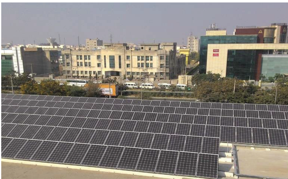
In November 2015, Bosch Limited commissioned a 600 kWp rooftop solar plant at Honda Motorcycle and Scooter Private Limited
