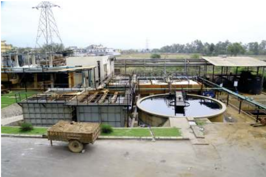
Effluent Treatment Plant
