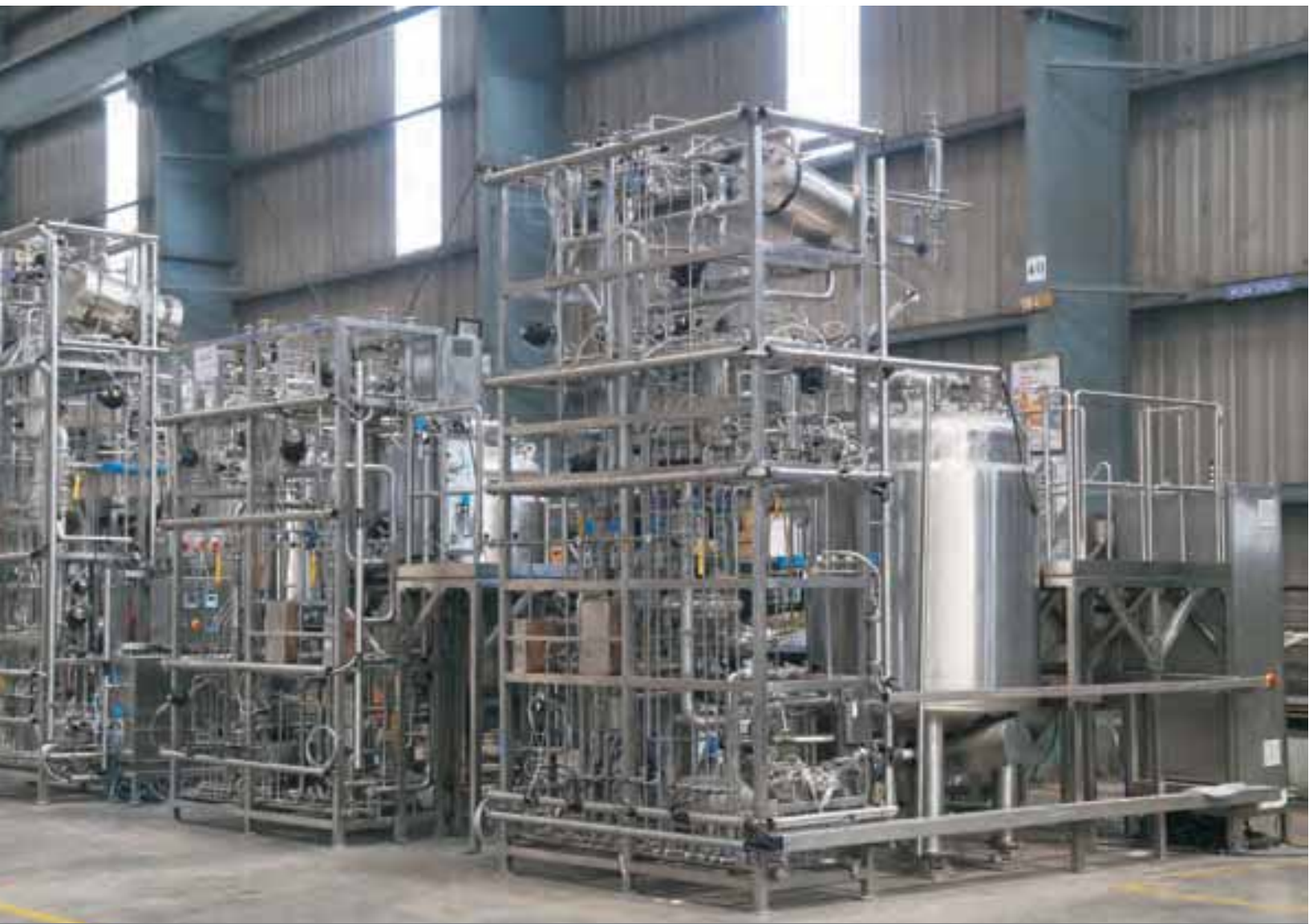
Skid mounted pharma system engineered and manufactured by Praj HiPurity Systems
