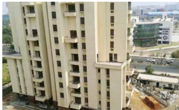
Construction of residential accommodation for NHAI staff at Pocket B5, Sector 17, Dwarka, New Delhi
