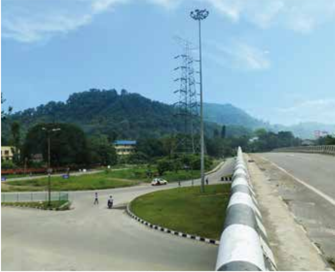
Two-laning to four-laning of Sonapur to Guwahati section of NH37 in Assam
