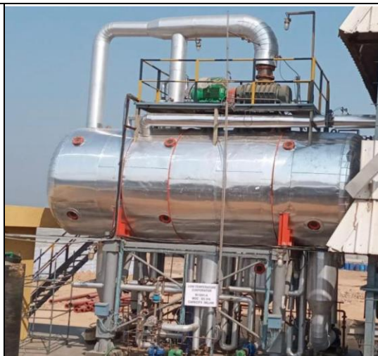
MVR_waste water treatment facility
