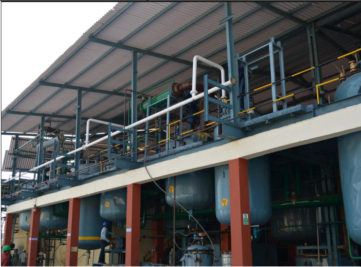
Reactors in Plant 3
