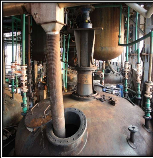
Machinery Name: C4 75KL Location In Plant: Main Plant Capacity: 75000LTR
