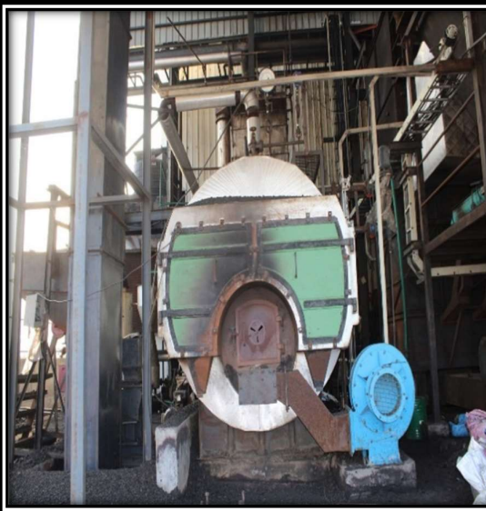
Machinery name: Coal fire boiler Location in plant: Hot air generator Capacity: 2000KGS Use: Boiler to Provide Steam
