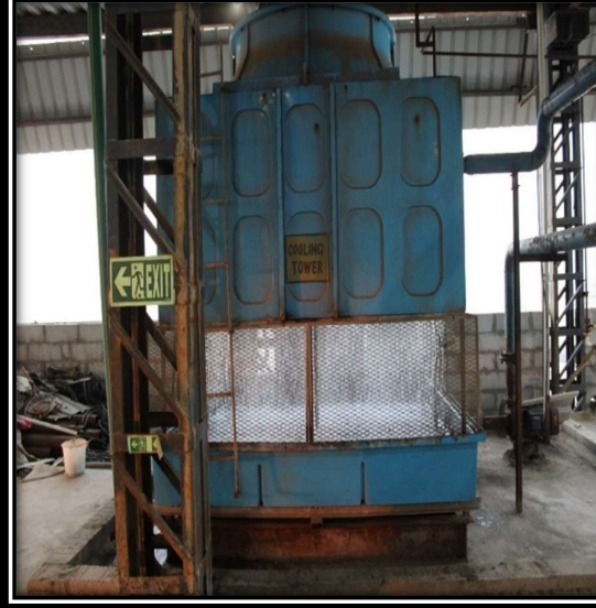
Machinery name: Cooling tower Location in plant: Main plant
