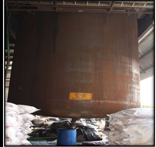
Machinery Name: C2 75KL Location In Plant: Main Plant Capacity: 75000LTR
