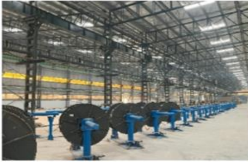
Phase I Furnace Equipments
