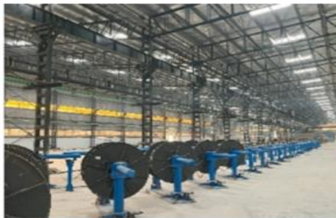
Phase I Furnace Equipments
