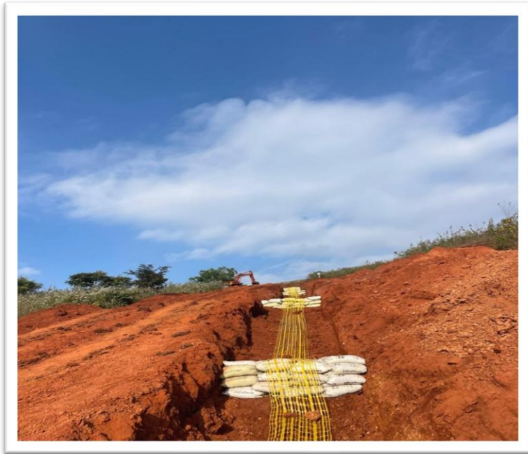
Slope Protection work in Hilly Portion of the 12" * 63 KM Gas Pipeline Project for Angul Srikakulam Pipeline Project, Part - B - Section IV, in Laxmipur, Odisha
