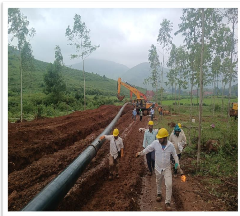
Lowering of 12" Dia * 63 KM Gas Pipeline for Angul Srikakulam Pipeline Project, Part B - Section IV, for NALCO, in Korapur, Odisha
