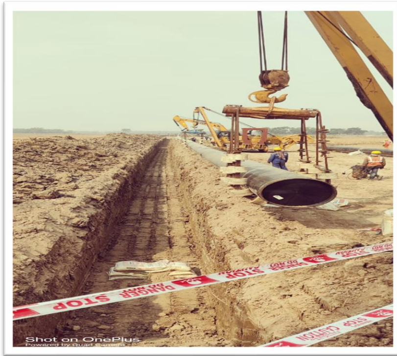
Lowering activity for 26" Dia * 142 KM Pipeline Project, for Paradip Numaligarh Crude Oil Pipeline Project, in Belda Area, West Midnapur, West Bengal
