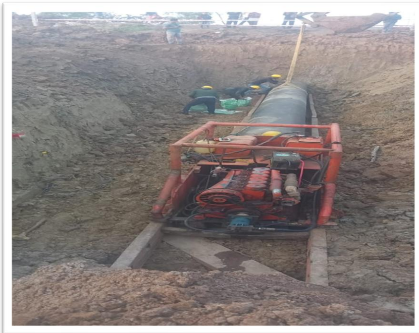
Thrust Boring for the National Highway Crossing of 32" Casing Pipe for the installation of 26" Dia * 142 KM Pipeline Project for Paradip Numaligarh Crude Oil Pipeline Project for Numaligarh Refinery Limited (NRL) in West Midnapur, West Bengal
