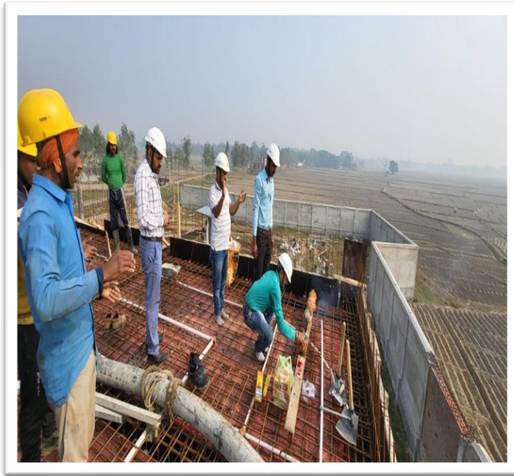
Start of concreting work for the slab of sectionalizing Valve (SV17) for the 26" Dia * 142 KM Paradip Numaligarh Refinery Limited (NRL), near Chandrakona, West Bengal
