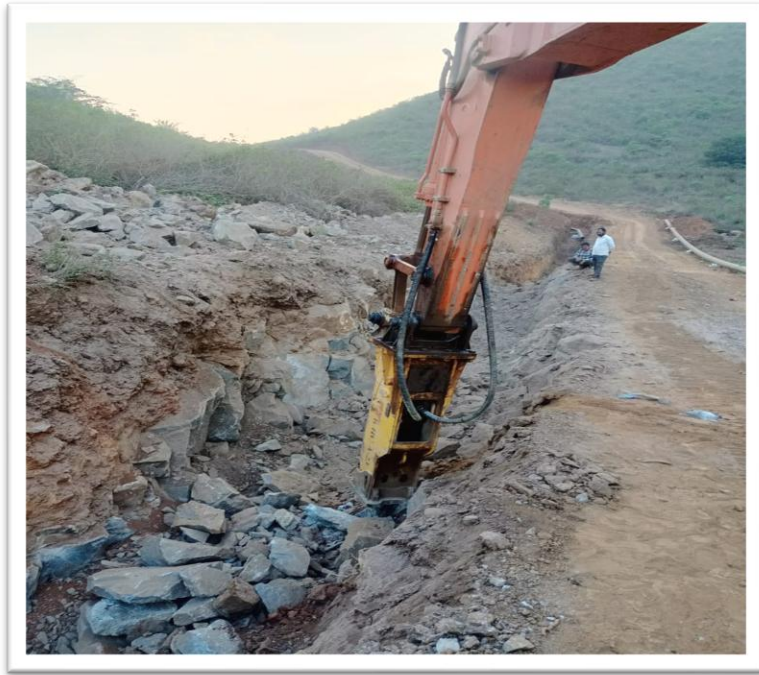
Trenching in rocky area, for the 12" * 63 KM Gas Pipeline for Angul Srikakulam Pipeline Project, for NALCO, near Laxmipur, Odisha
