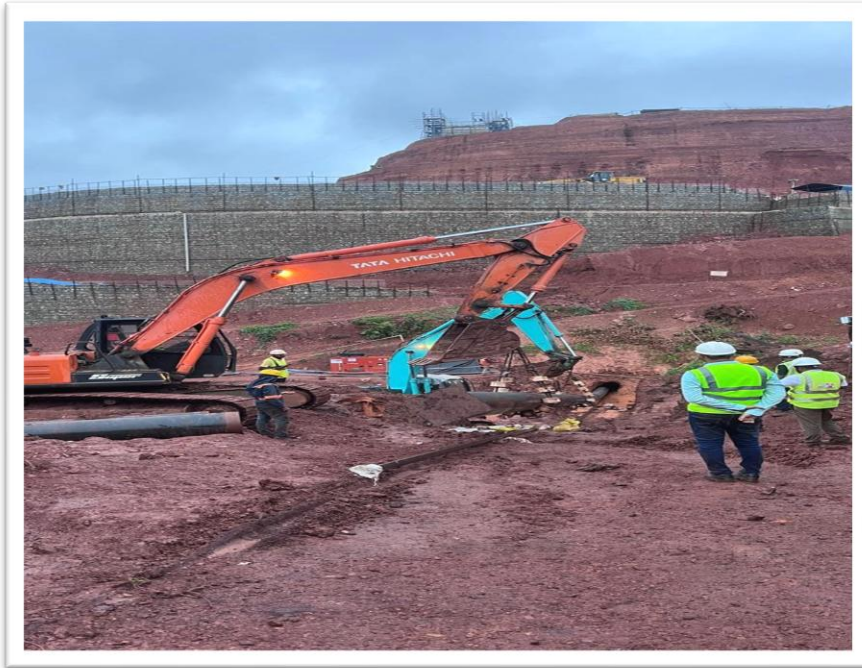
Horizontal Directional Drilling (HDD) of Hill Portion Crossing at 59 m depth (from top of the Hill) for the 20" Slurry Pipeline inside Sagasahi Mines for Arcelor Mittal - Nippon Steel (AMNS) in Barbil Area, Odisha
