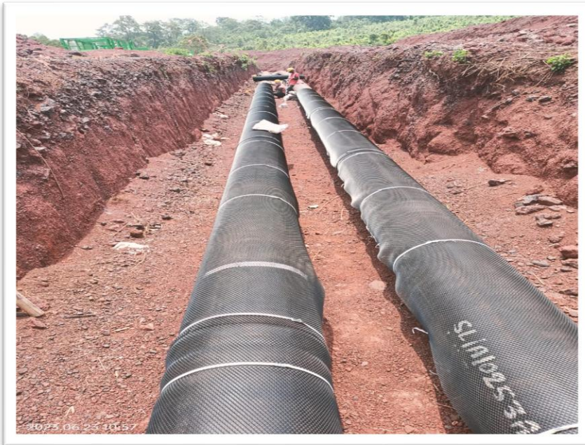
Pipeline Installation works in Rocky Area, with Rockshield protection, for the 2 Nos * 20" Dia * 30 KM Slurry & Return Water Pipeline from Sagasahi to Dabuna, for Arcelor Mittal - Nippon Steel (AMNS), in Odisha
