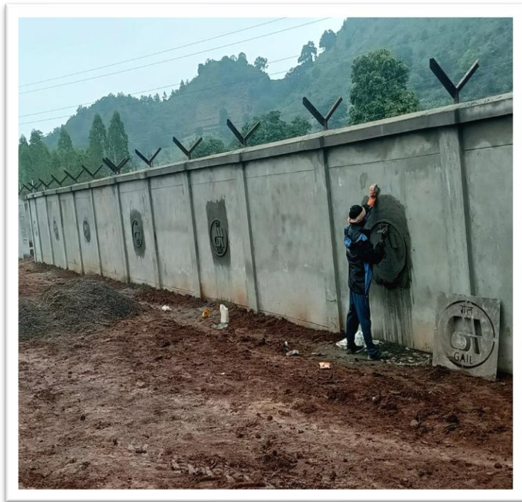
Construction of remote operated – sectionalizing Valve Station (SV01N) for Angul Srikakulam Gas Pipeline Project of GAIL, for NALCO, in Reygada, Odisha
