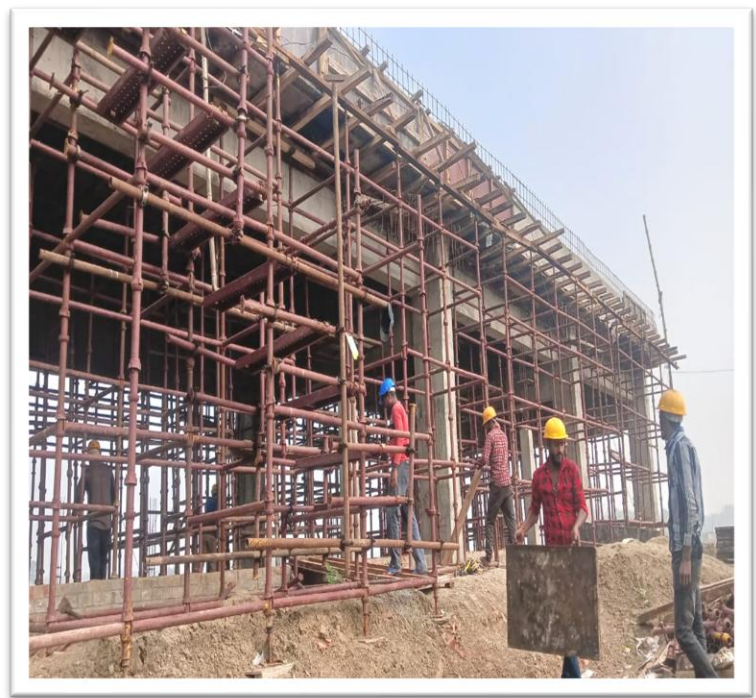
Construction of sectionalizing Valve Station (SV16) for the 26" Dia * 142 KM Paradip Numaligarh Crude Oil Pipeline Project for Numaligarh Refinery Limited (NRL), near Kharagpur, West Bengal
