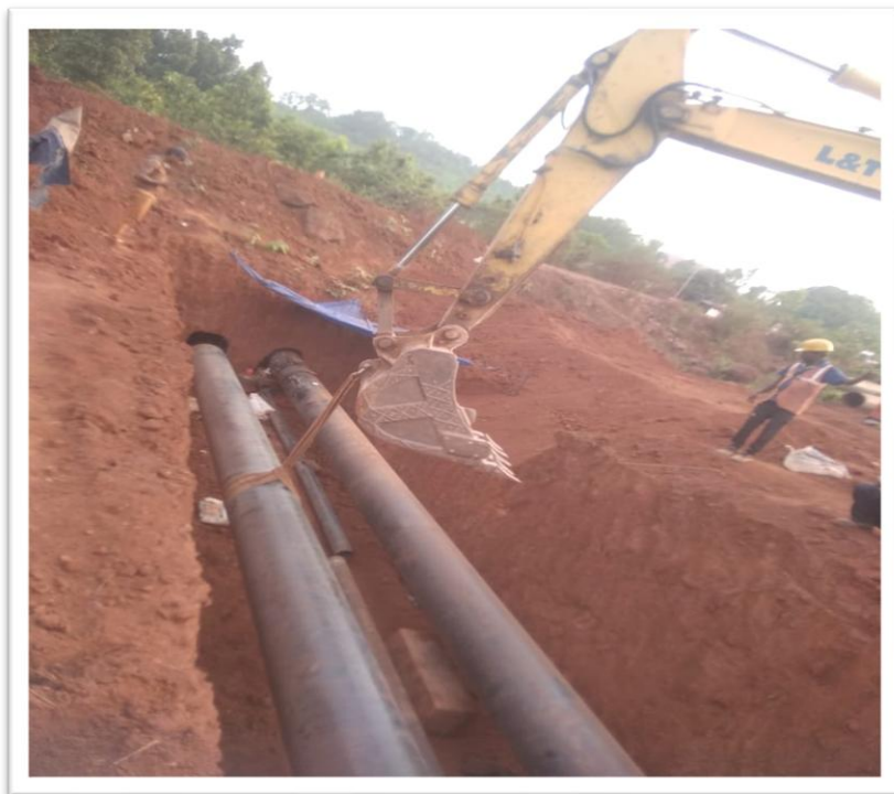
Shallow HDD Crossing of Road section of the 2 Nos * 20" Dia * 30 KM Slurry & Return Water Pipeline from Sagasahi to Dabuna, for Arcelor Mittal - Nippon Steel, in Odisha
