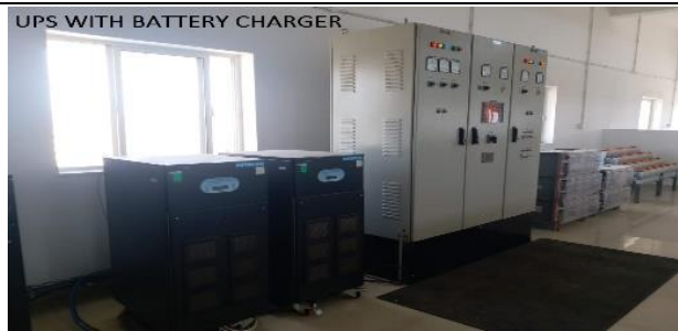
UPS with battery charger
