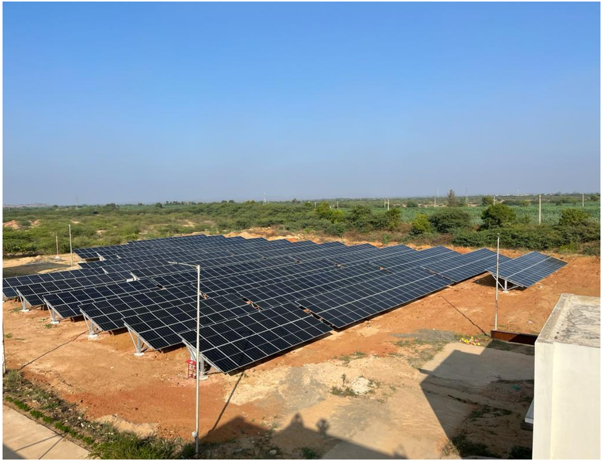
Ground Mounted Project
