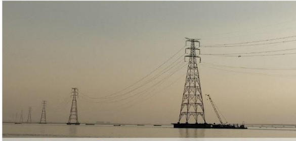
400 kV Padma River Crossing Transmission Line, Bangladesh
