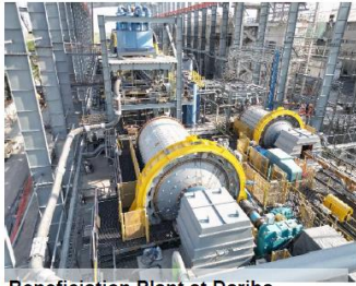
Beneficiation Plant at Dariba, Rajasthan
