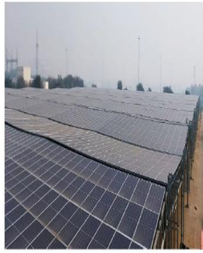
20 MW Solar Carport project, Haryana
