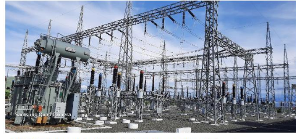
132 kV Air Insulated Substation, Papua New Guinea
