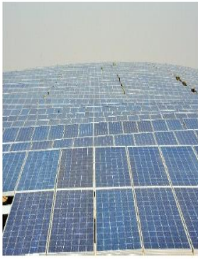
150 MWp Ground Mount Solar Project, Rajasthan
