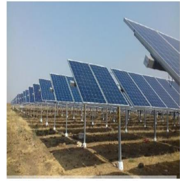
30 MW Tracker Based Installation, Andhra Pradesh
