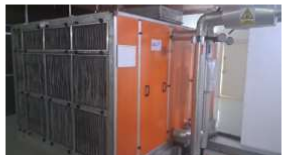
Typical AHU (part of Subject Property) on all floors of Subject Tower
