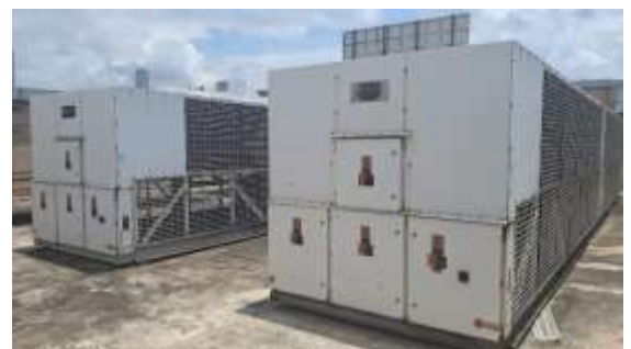
View of Chillers on terrace of Subject Tower
