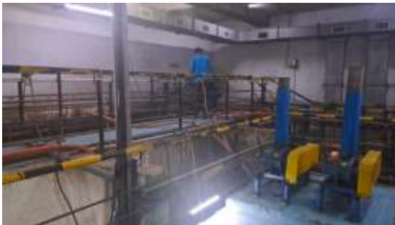
Internal View of STP in Subject Tower
