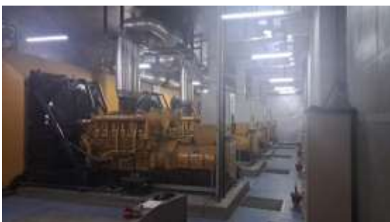
Internal View of DG Set Room in Subject Tower
