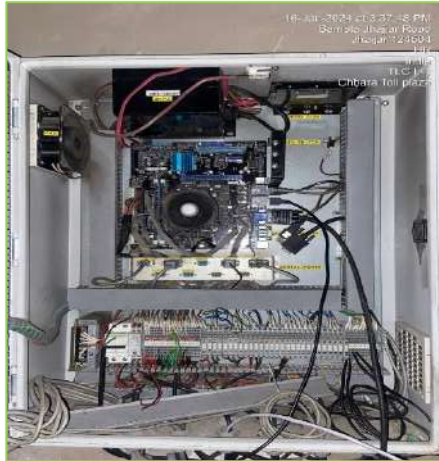
Figure 3-10: Toll Lane Controller at Tunnel
