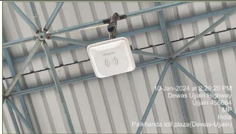
Figure 3-14: RFID ETC Transceiver installed on pole
