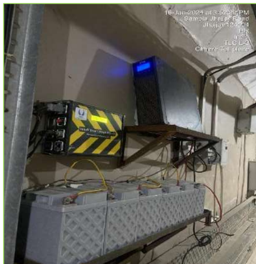
Figure 3-23: Lane UPS in Tunnel.
