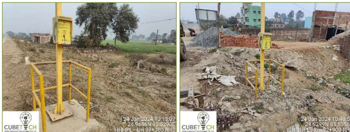
Figure 3-12: Emergency call box
