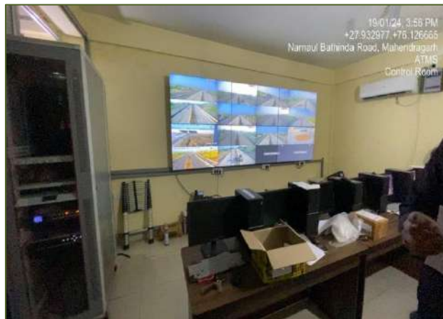
Figure 3-29: Workstations in ATMS control room.
