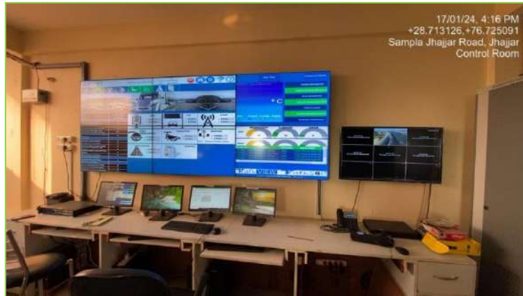
Figure 3-31: ATMS Control Room.
