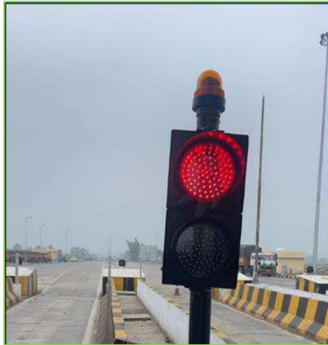
Figure 3-18: Lane Traffic Light (LTL)
