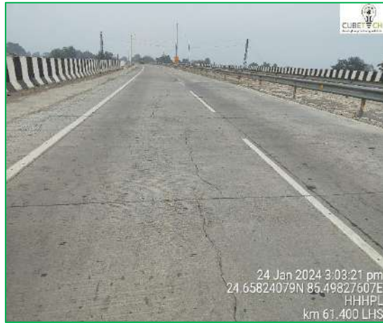
Figure: Longitudinal Cracks
