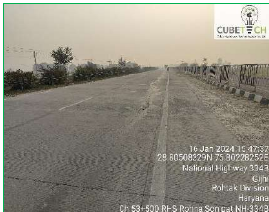
Figure: Longitudinal Cracks
