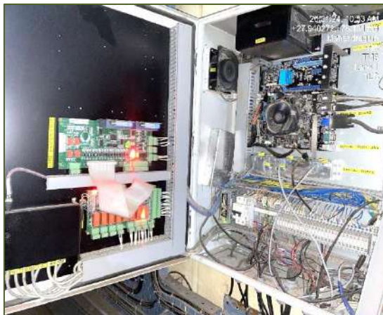
Figure 3-9: Toll Lane Controller inside Tunnel.
