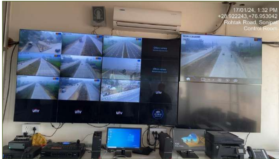
Figure 3-30: ATMS Control Room Equipment.
