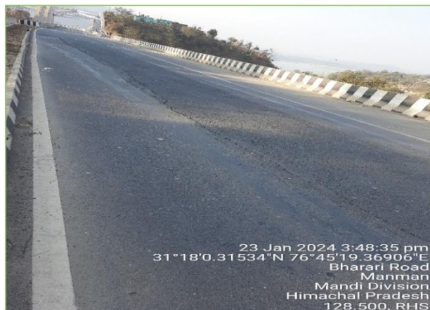
Figure: Longitudinal Cracks
