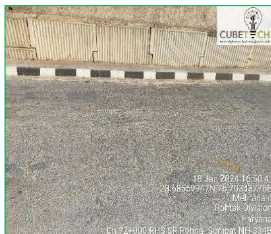
Figure: Alligator Cracks
