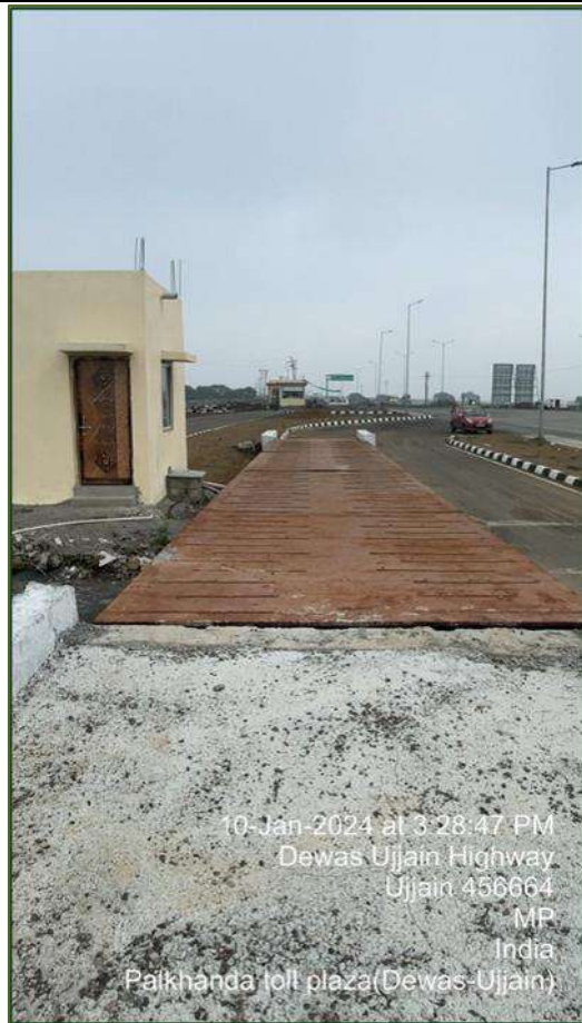
Figure 3-23: Static Weigh Bridge
