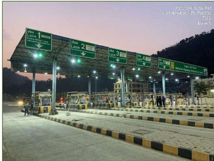
Figure 3-15: Over Head Lane Signal (OHLS).
