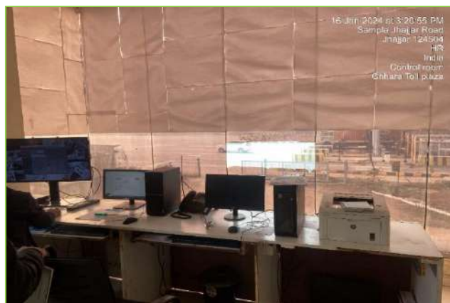
Figure 3-21: Workstations at Control room.
