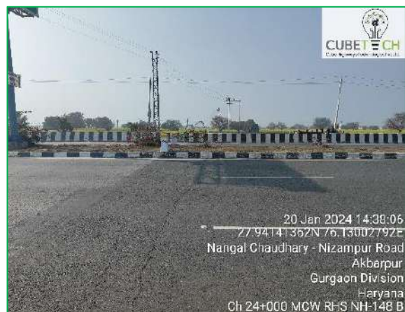
Figure: Transverse Cracks
