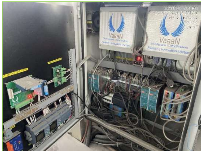
Figure 3-16: Toll Lane Controller inside Booth
