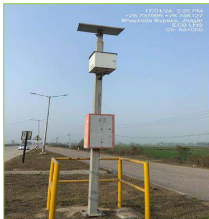
Figure 3-24: Emergency Call Box.
