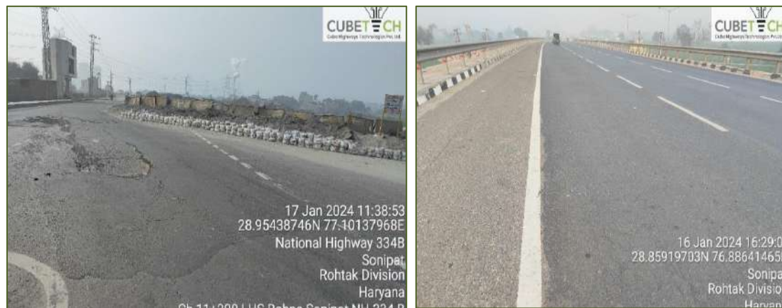
Figure: Alligator Cracks
