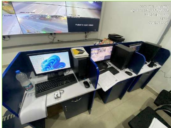
Figure 3-41: Workstations in ATMS control room.
