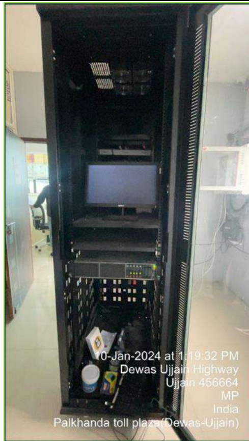
Figure 3-25: Server with rack.
