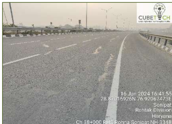
Figure: Longitudinal Cracks
