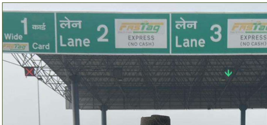
Figure 3-15: Over Head Lane Signal (OHLS).
