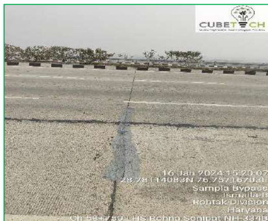
Figure: Spalling of joints
