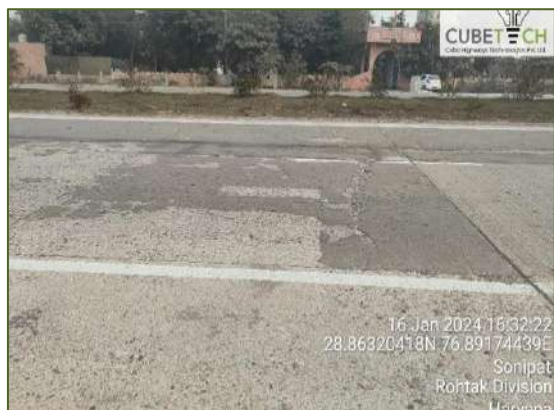
Figure: Tranverse Cracks
