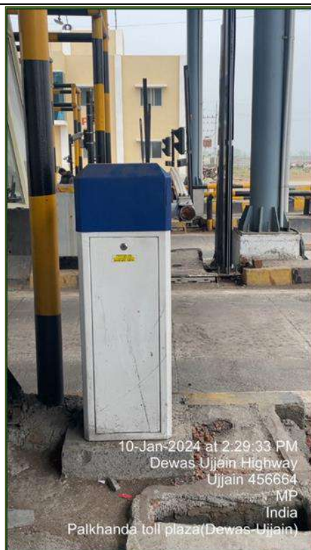
Figure 3-17: Automatic Lane Barrier
