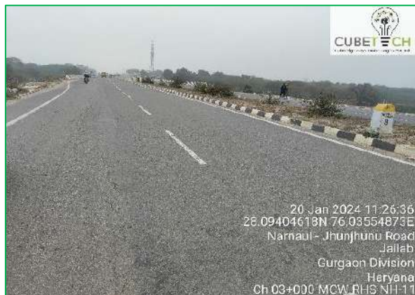
Figure: Longitudinal Cracks
