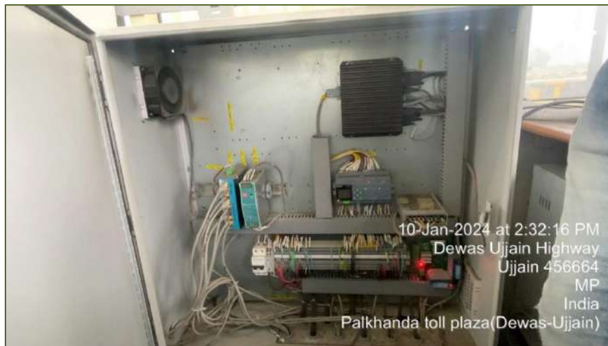
Figure 3-15: Lane Controller at Toll Booth
