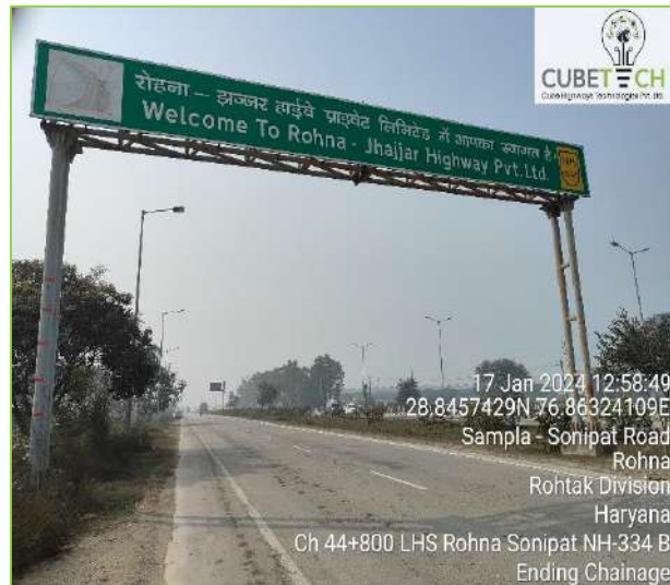
Figure 3-5: Overhead & Cantilever Gantry boards
