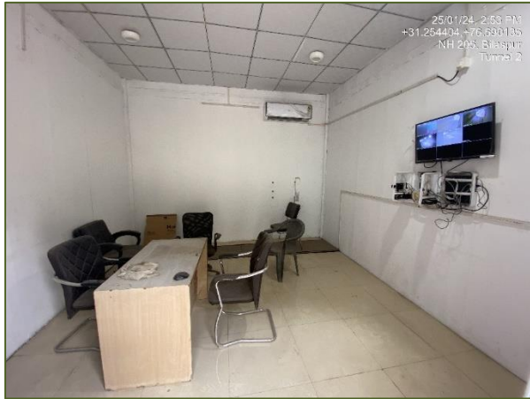
Figure 3-47: Tunnel-2 Control Room.
