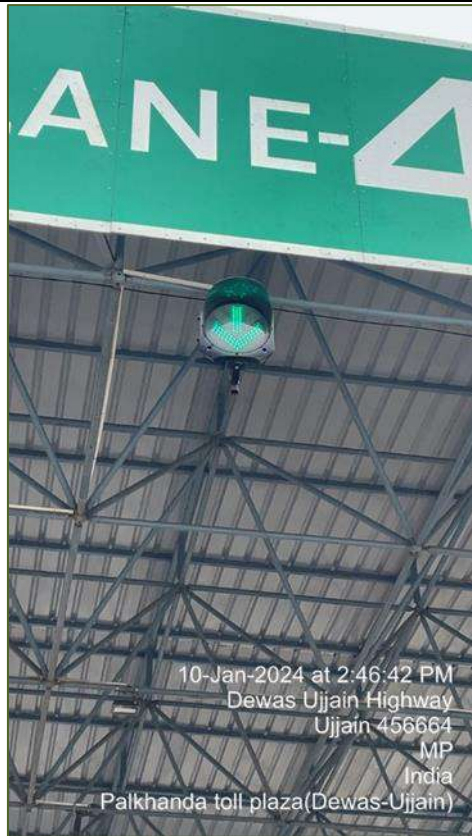
Figure 3-20: Over Head Lane Signal (OHLS)
