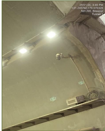
Figure 3-44: Tunnel-1 PTZ Camera.
