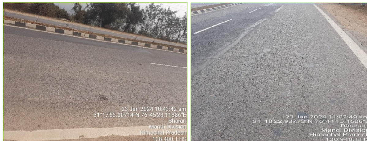
Figure: Alligator Cracks
