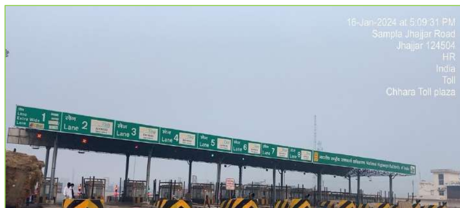
Figure 3-16: Over Head Lane Signal (OHLS).
