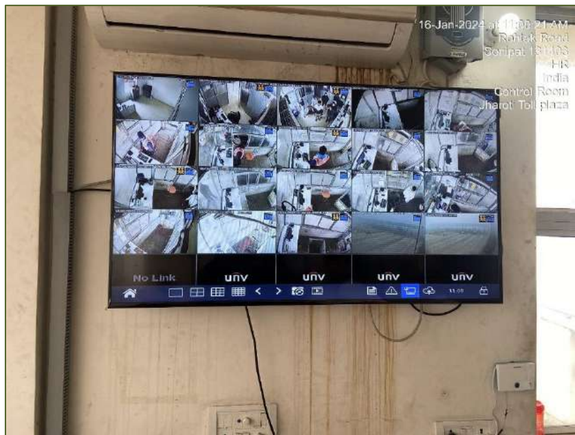
Figure 3-20: CCTV screen at the Toll Plaza Control Room.
