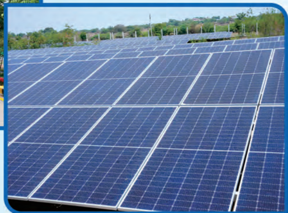
Installation of 1 MW solar power unit
