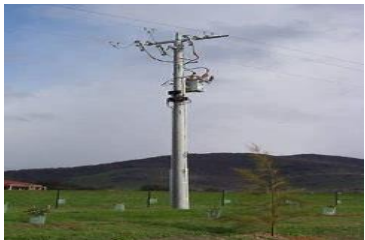
Power Distribution Poles
