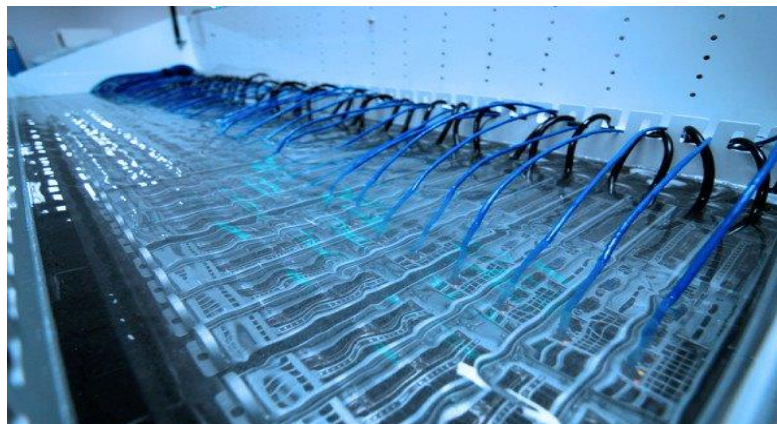
DATA Centre Cooling
