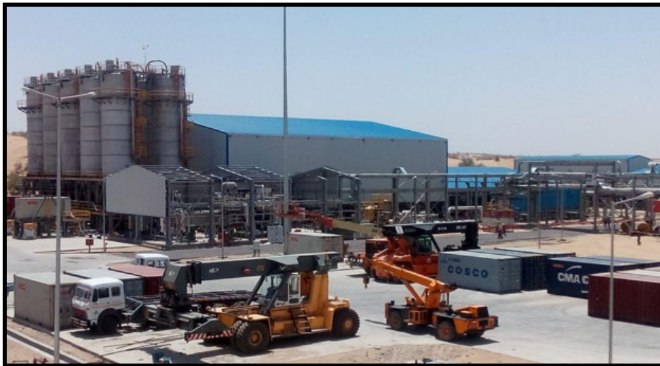
Central Polymer Facility – Silos and Trains
