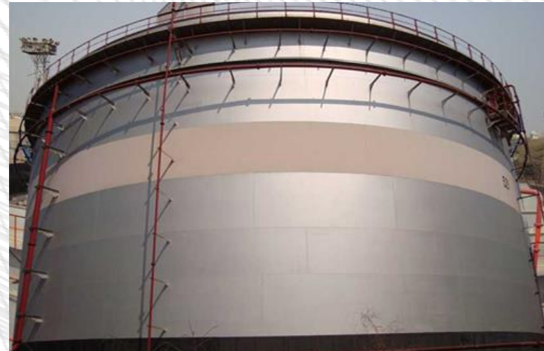
Floating Roof Tanks
