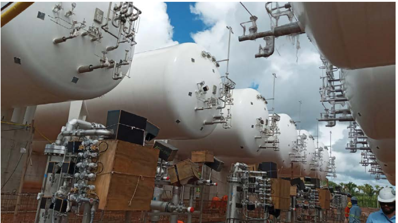
Designed, manufactured and erected 311 M 3 Liquid Hydrogen tank in South Korea. This has been done for one of the biggest hydrogen installation facilitating mobility application.
