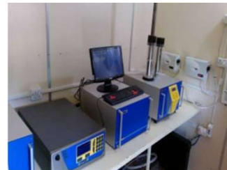
Online Continuous Air Quality Monitoring Station
