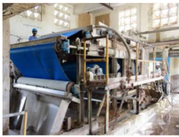
Sludge Handling - Paper
