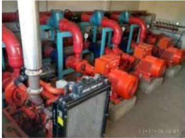
Fire Hydrant Pumps
