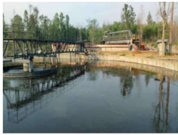
Secondary Clarifier - Pulp
