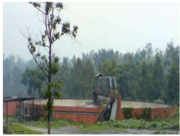
Primary Clarifier - Pulp
