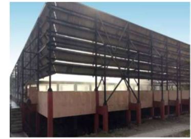
Mist Cooling System
