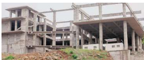
The under-construction Tribal Museum in Garudeshwar where two tribal youths were allegedly assaulted to death last week. Bhupendra Rama
