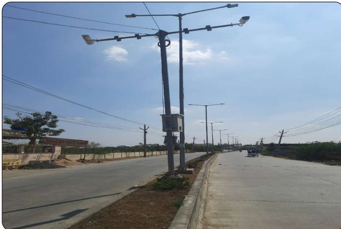
Fibre Network & Cloud Surveillance system at Markapur, Prakasam District, Andhra Pradesh
