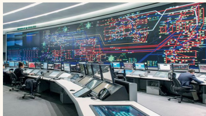
State of the art IT integrated infrastructure
