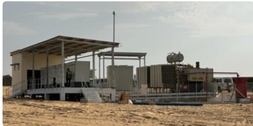
Inverter Control Room
