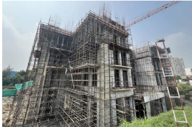
Tower 3 - As on 25 th Oct 2024 – Third floor slab is completed, and 4 th floor is work in progress
