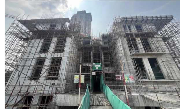
Tower 2 - As on 25 th Oct 2024 – Third floor slab is completed, and 4 th floor is work in progress
