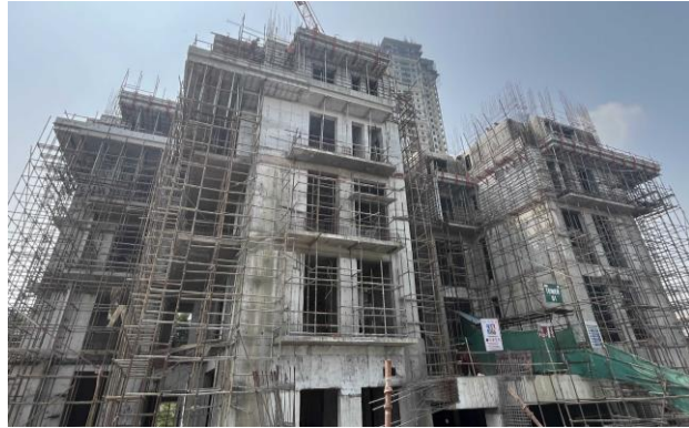
Tower 1 - As on 25 th Oct 2024 – Fourth floor slab is completed, and 5 th floor is work in progress
