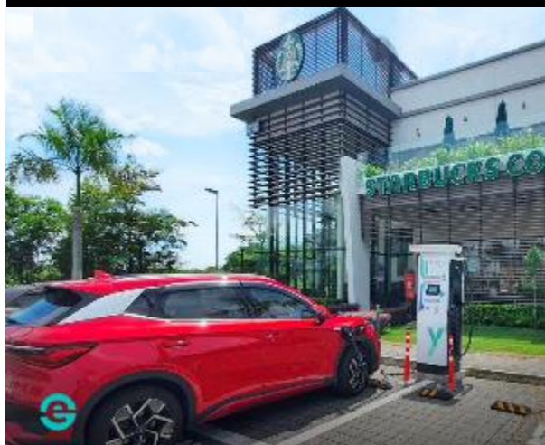
Heavy-duty DC charger installation at Starbucks Malaysia
