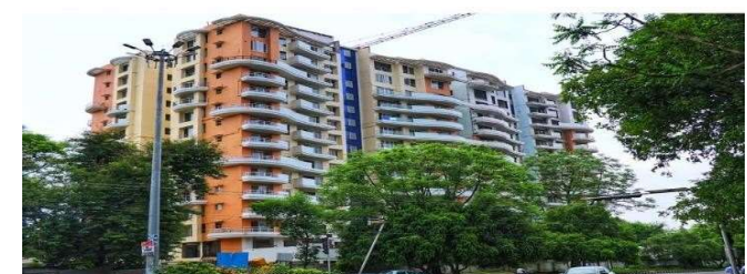
Construction of 96 flats at Tulsi Tower, Bhopal for MP Housing & Infrastructure Development Board
