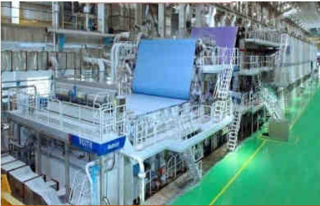
FINISHED PAPER – 1,82,400 TPA
