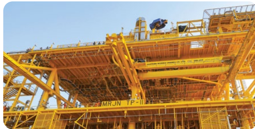
Saudi Aramco Marjan II - Offshore Platform project at Hazira, Surat by Asian Paints PPG (Contractor - L&T Hydrocarbon)
