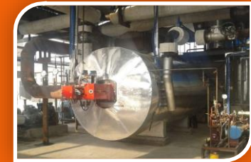
3.5 MW Thermal Oil Heater for Biscuit Baking
