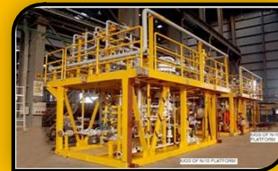
Instrument Utility Gas Drying Systems
