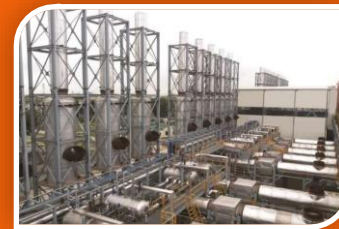
16 MW Waste Heat Based Power Plant for 200 MW IPP
