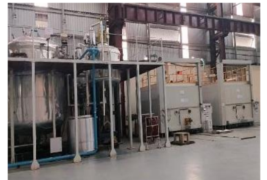
VPI Plant with Oven
