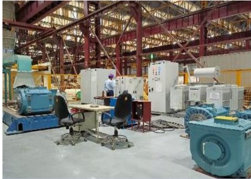
Traction Motor Testing facility
