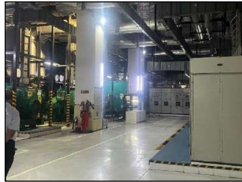
View of LT Room
