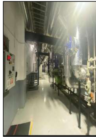
Internal View of Plant Room Tower 4, 5 & 6
