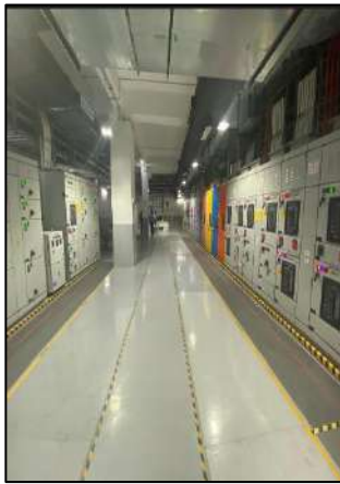
View of DG Room Tower 4 ,5 & 6
