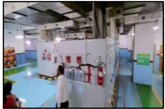
View of Electrical room
