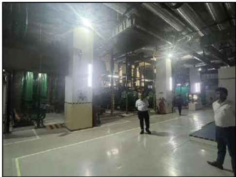
View of DG Room
