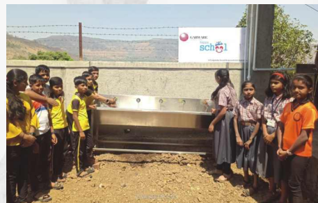
Improving hygiene practices among students by installing a handwashing facility at Zilla Parishad Prathamik Kendrashala, Hatgeghar, Satara
