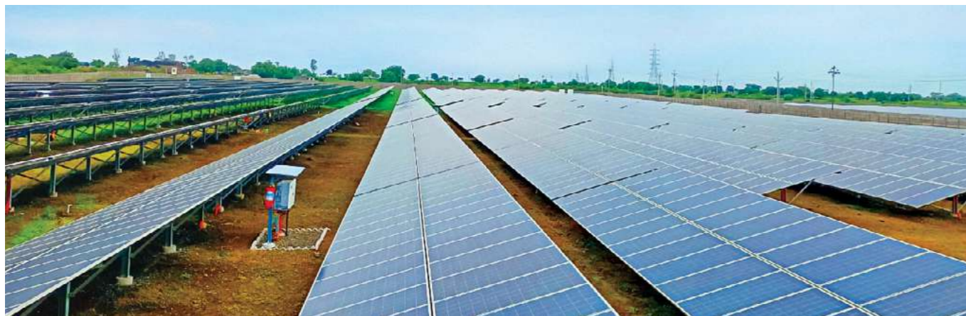
Solar power plant @ Partur, Maharashtra
